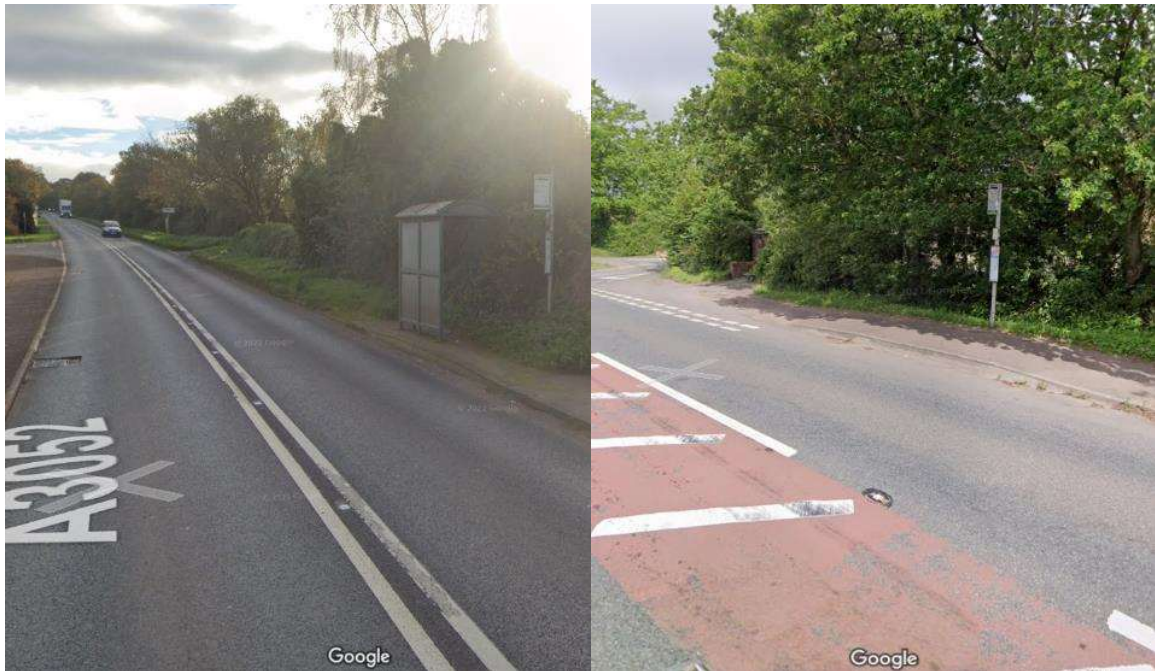
Figure 5.7: Inadequate Bus Stops along A3052
